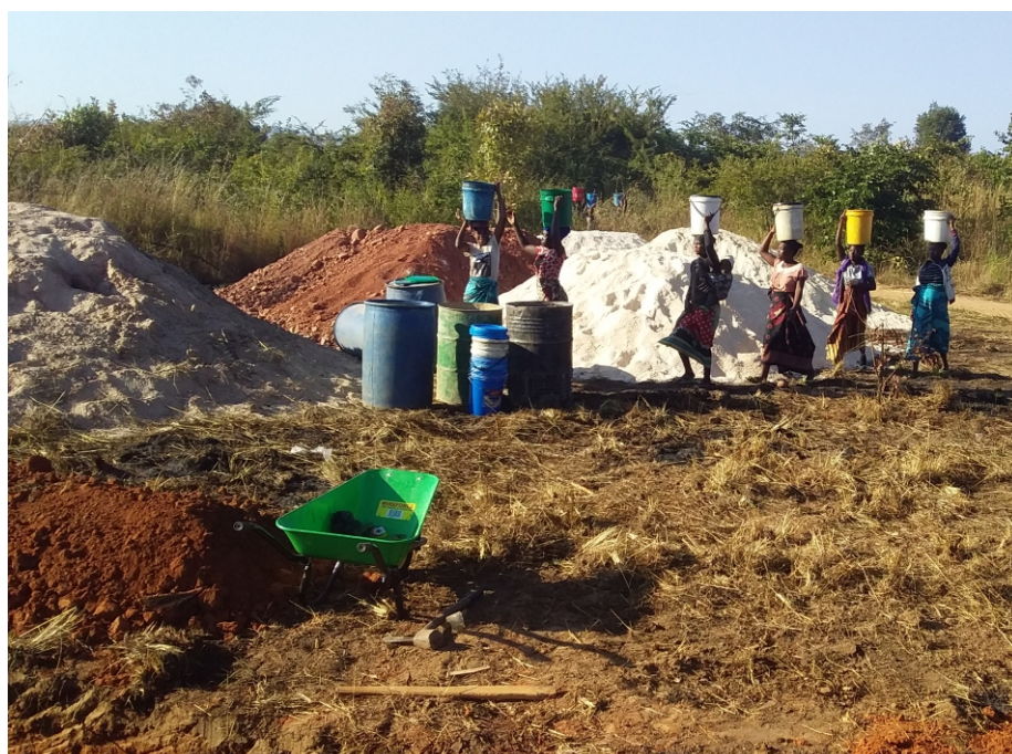
Women participating in the construction of their community seed bank; community participation is essential in ensuring sustainability of projects.
